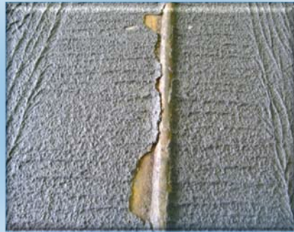
Welds see more impact
